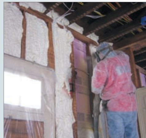
On top of the rain screen, we installed \frac{1}{2} -inch rigid foam board, then sprayed foam into the wall cavity.
